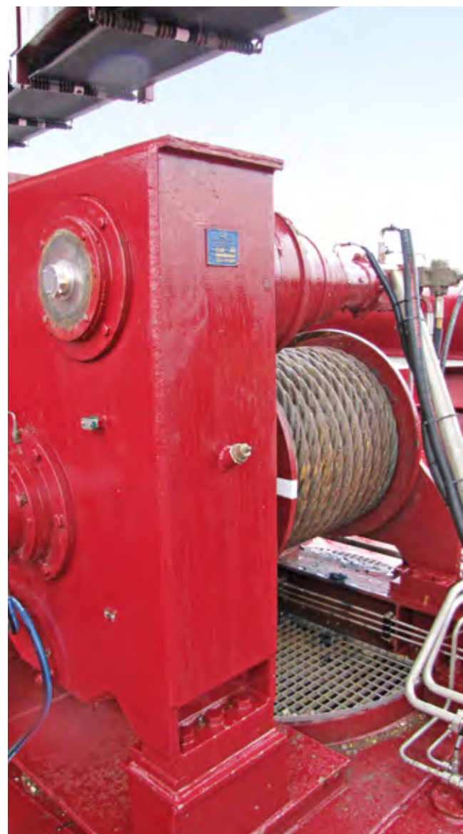
Three of these winches guide the suction pipe, at top left, an encoder detects the rotation of the shaft.
