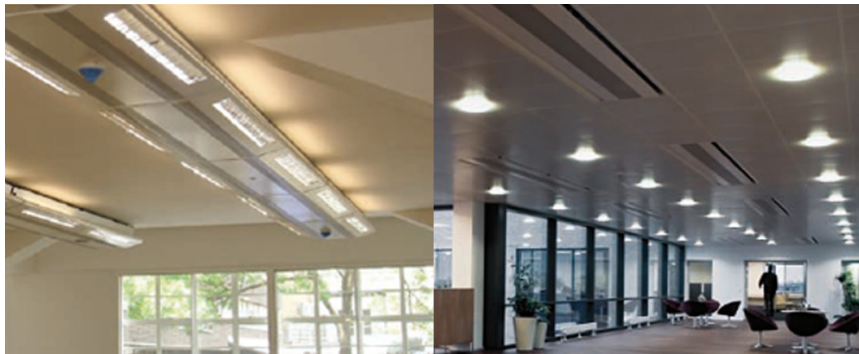
Figure 12. Examples of active chilled beam installations
