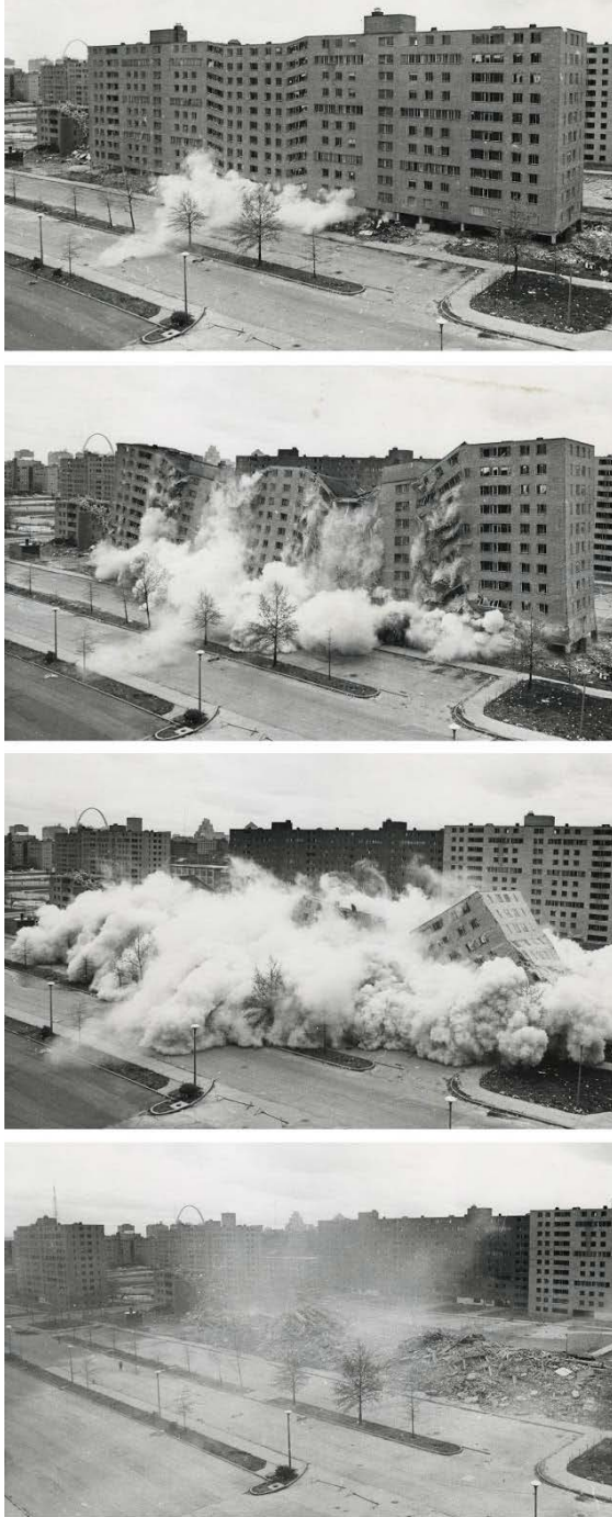
Figure 4-10. April 1972. The second, widely televised demolition of a Pruitt-Igoe building that followed the March 16 demolition. Image: U.S. Department of Housing and Urban Development.
