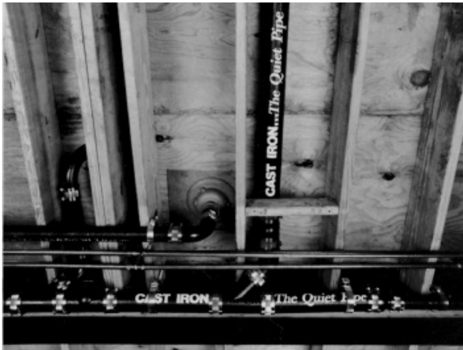
Figure 1—Cast Iron in Residential Application.
