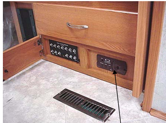
LP Gas Alarm
