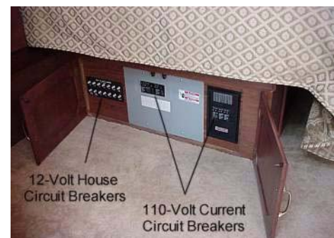
House 12V Breakers
