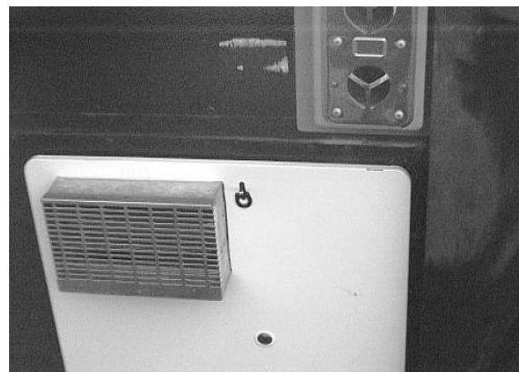
Water Heater Service Access Panel
