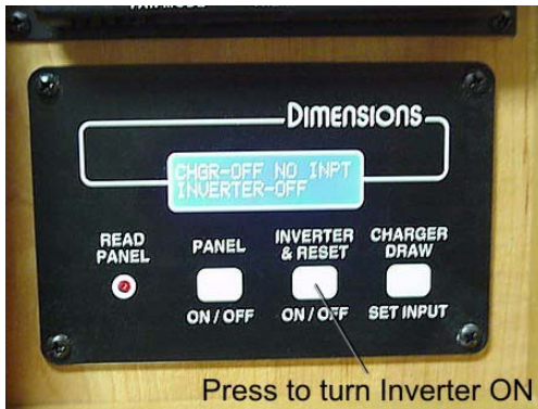
Inverter Charger Control Panel
