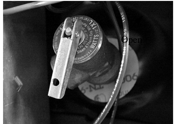
Lift handle straight out to open P-T valve.
