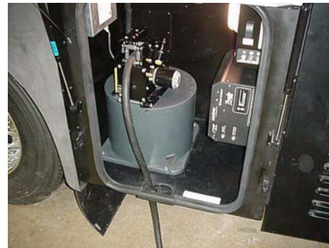
Inverter Charger Unit Location in shoreline compartment
