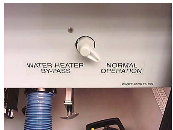
Water Heater By-Pass Valve (Typical)
