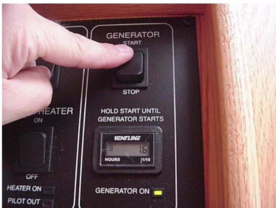
Generator Switch and Hourmeter
