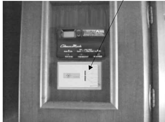
Power Ventilator Thermostat - Galley
