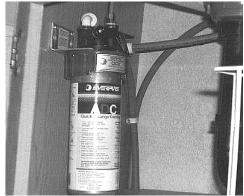
Water Filter Assembly - Below Galley Sink
