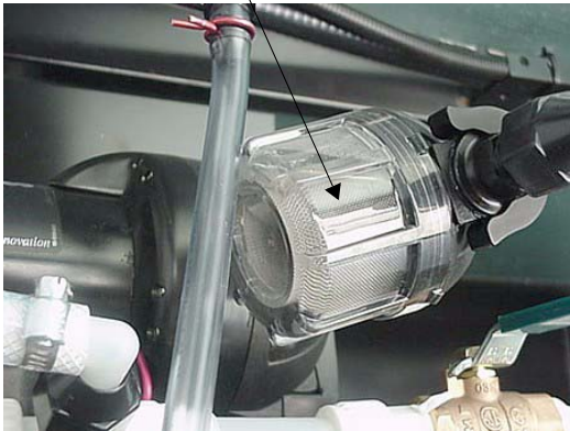
Water Pump Filter
