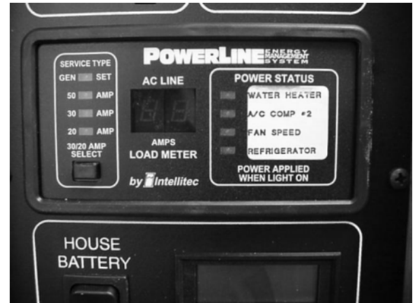
EMS Display on OnePlace Monitor Panel
