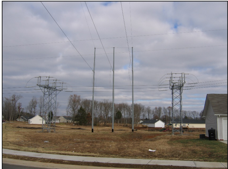
Photo 2-3. Example of switch structures and associated 3-pole transmission structure at a transmission line tap point
