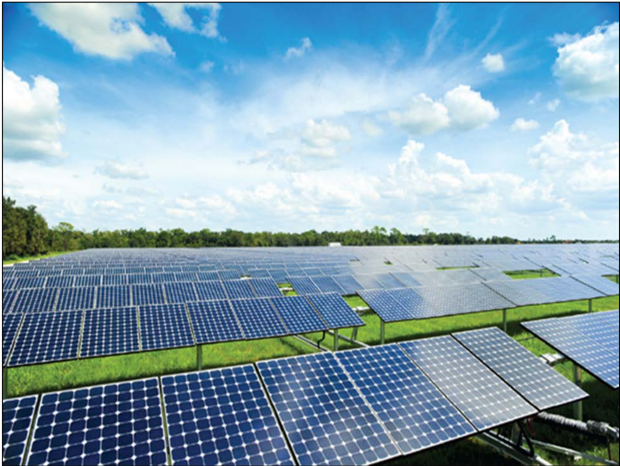
Photo 3.5-5. Single-axis, tracking photovoltaic system with panels close to maximum tilt
