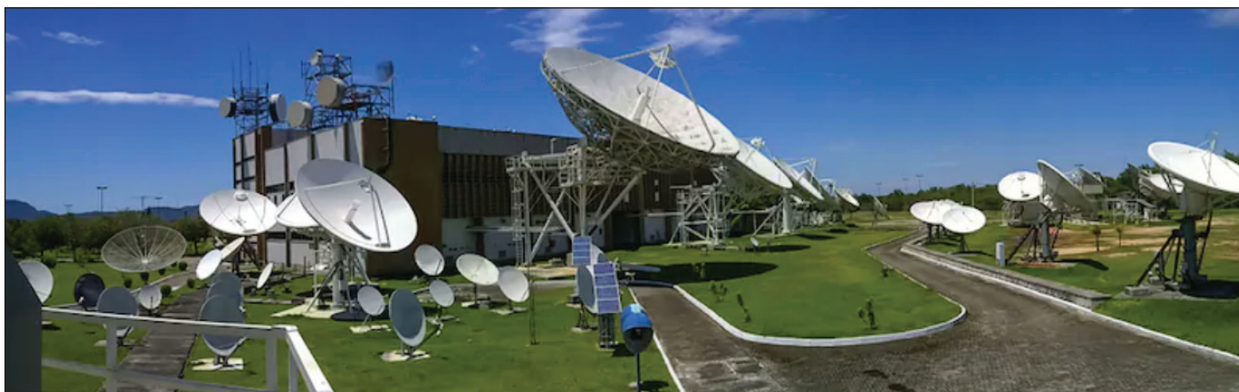
Figure 1. Satellite Earth Station
