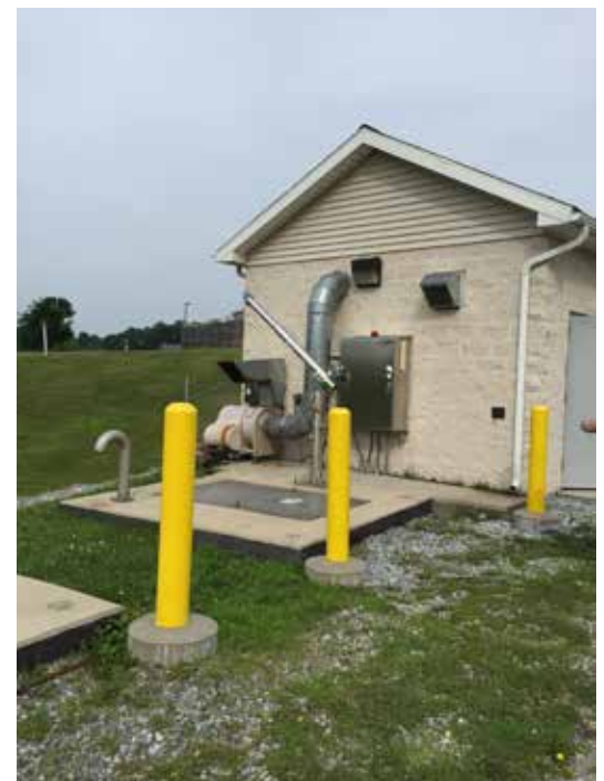
Chester County Prison pump station
