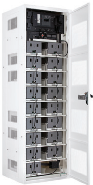
Lithium-ion battery systems provide a reliable and flexible solution that ensures 24/7 system uptime
