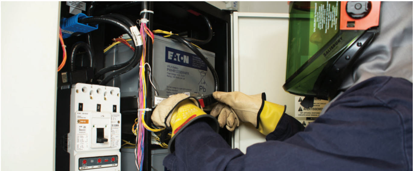
Appropriate personal protective equipment is essential when working on batteries or any UPS equipment
