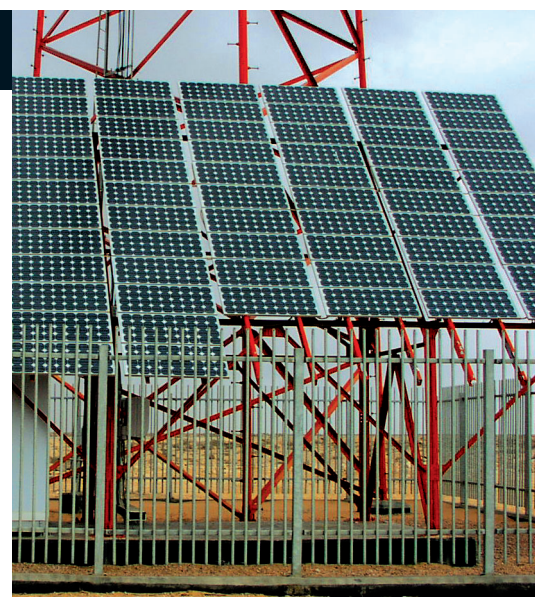
5% of Vodafone's base stations in Greece have solar panels, with 111 solar base stations in total
