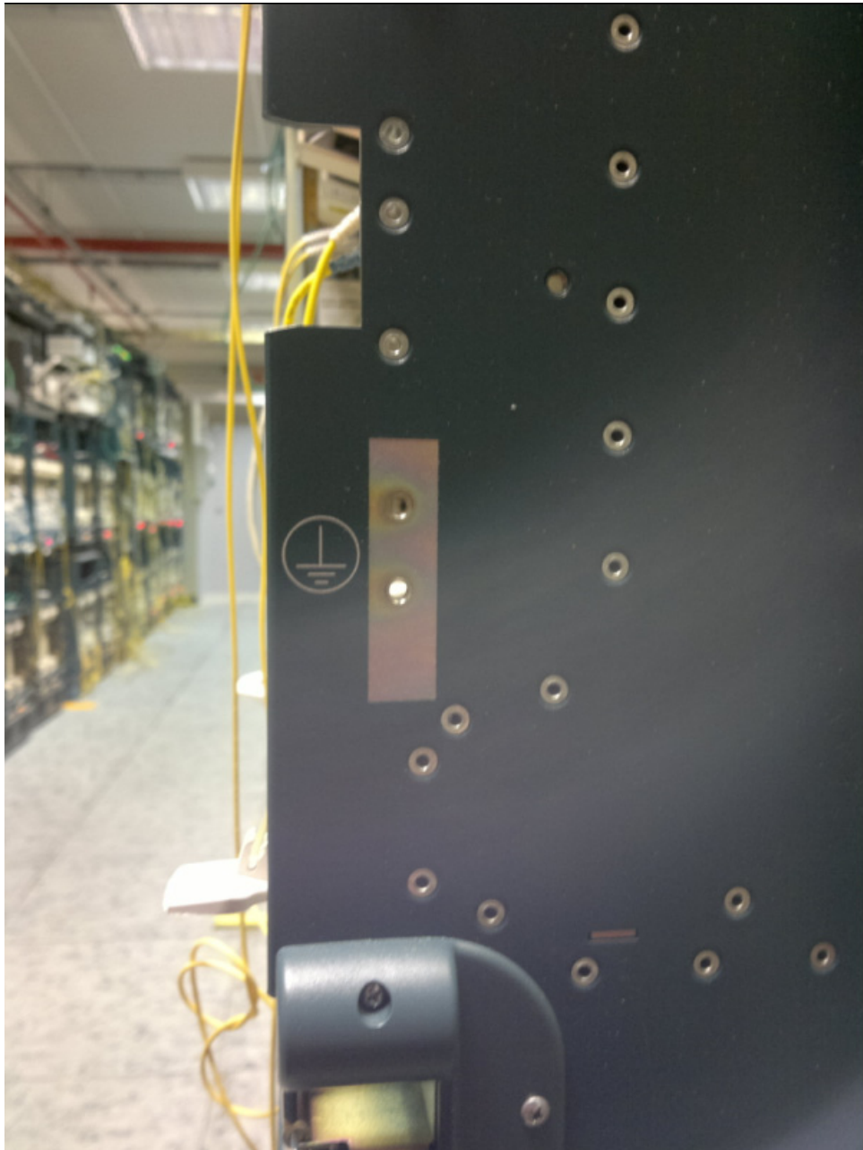
Figure 2-13 Missed System (NEBS) Grounding on a Cisco ONS 15454
