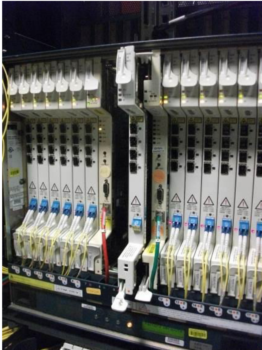
Figure 2-25 Card not Properly Inserted in the Chassis
