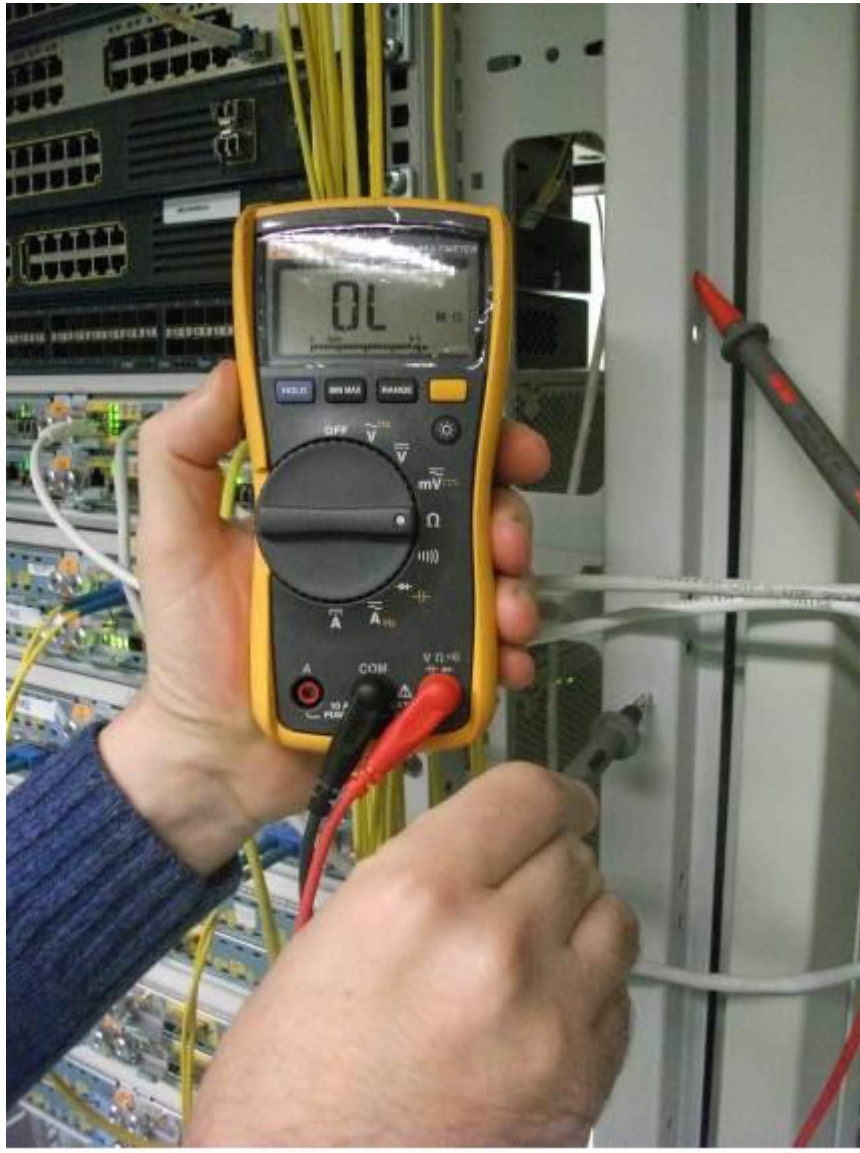
Figure 2-22 Non-conductive Paint on a Rack
