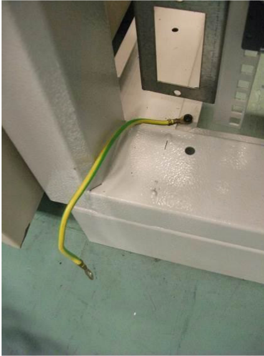
Figure 2-11 Rack Grounding Cable not Connected to the Grounding Bar
