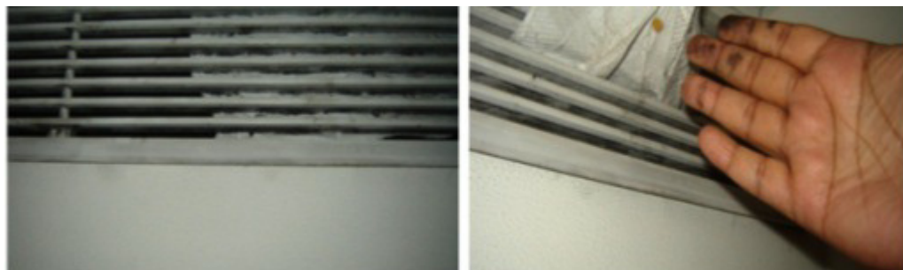
Figure 3-13 Clogged Air Conditioner Duct
