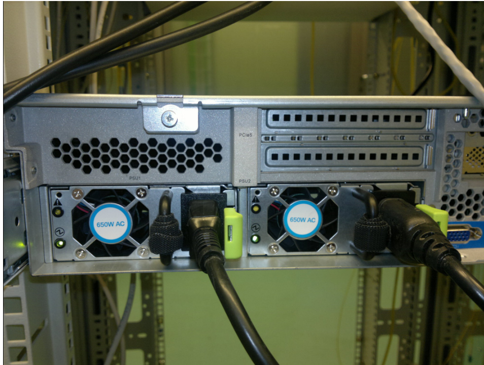
Figure 2-32 Equipment Powered by Two Separate Power Supplies (one redundant)
