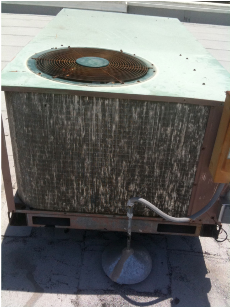
Figure 3-20 Air Conditioner not Working at an Installation Site (No Periodic Maintenance)
