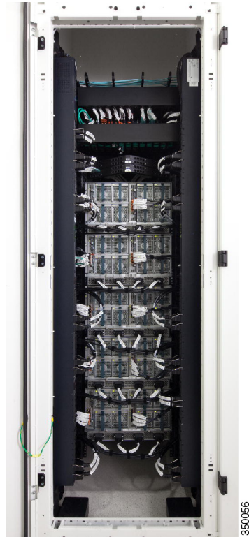
Figure 2-39 Main Door of a Closed Cabinet Removed to Improve Airflow
