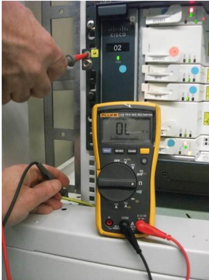
Figure 2-15 Ineffective Metal-to-Metal Contact between Cisco Chassis and Installation Rack
