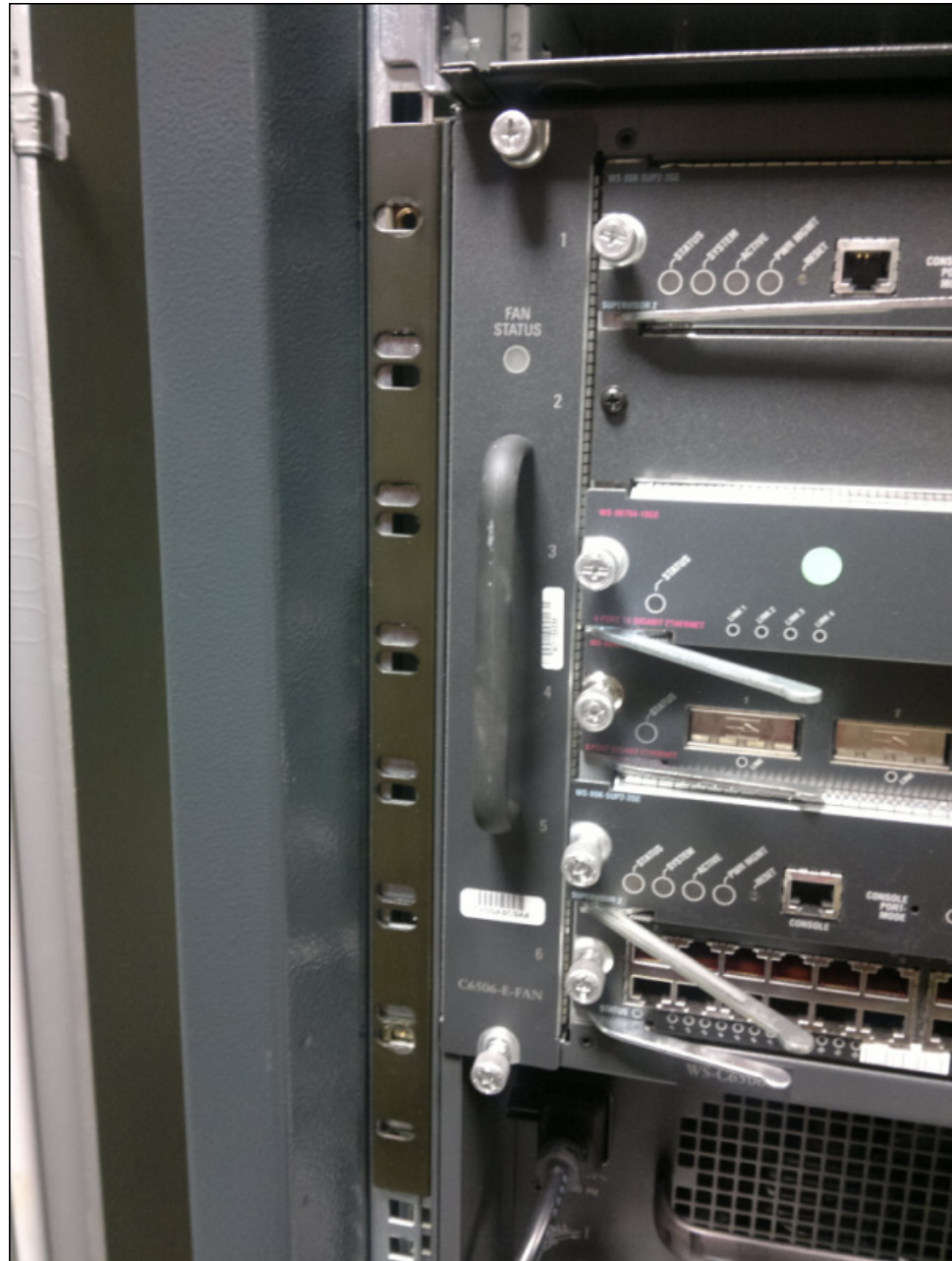
Figure 2-31 Missing Screws when Connecting Cisco Data Networking Equipment to the Rack
