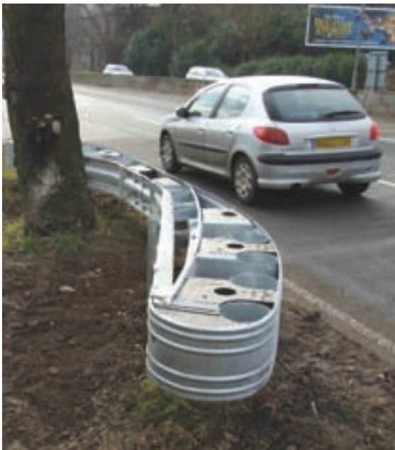
A tree protection system in operation
