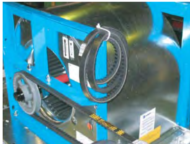
SPARE FAN BELT (Attached to Fan)
