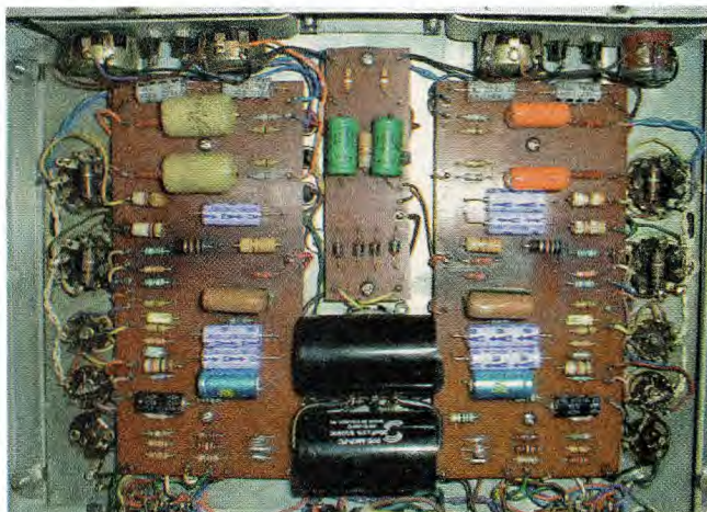
Photo 2: Layout under the chassis. There are three PCBs, one each for the right and left channels and a small one (centre) for the silicon HT rectifiers and the bias supply components.
