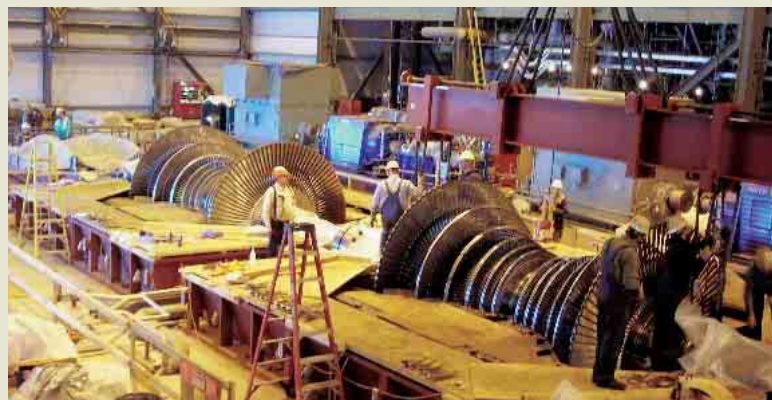
Steam turbine for thermal power generation in North America
