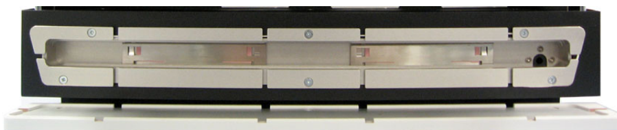
Fig. 19: View into the column compartment
