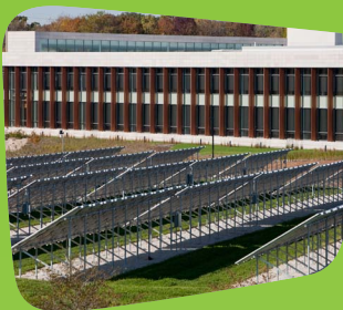
The solar photovoltaic field at Johnson Controls Corporate Headquarters in Glendale, WI
