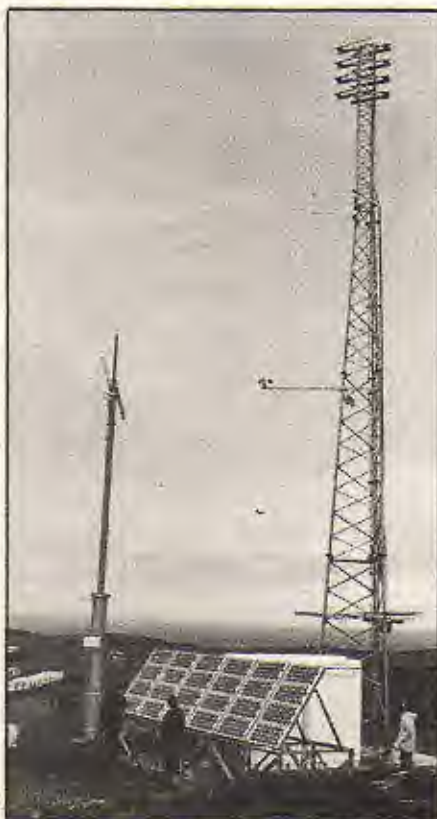
The wind and sun powered transmitter installed by the IBA in Bossiney, Cornwall.
