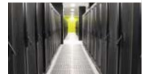
New machine room at the Fujitsu Tatebayashi System Center
