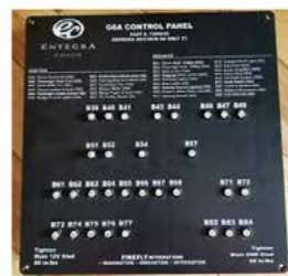
GFCI Breaker Panel
