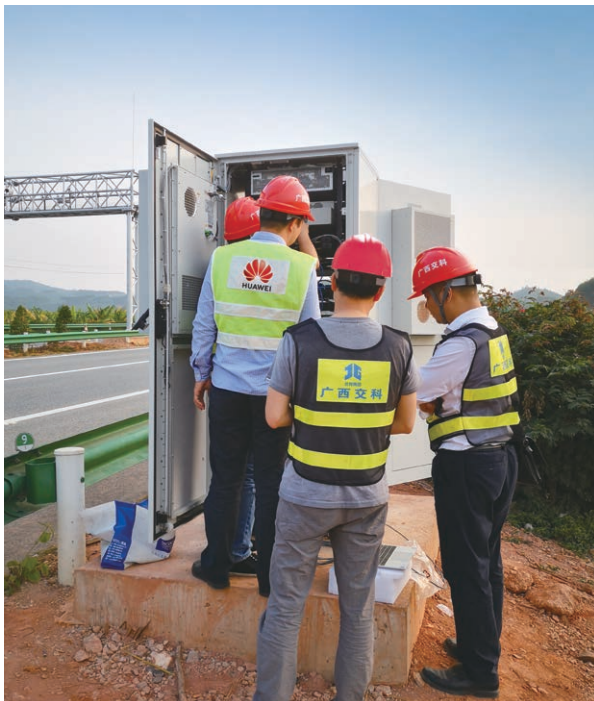
Site installation for an ETC gantry system in Guangxi Province, China
