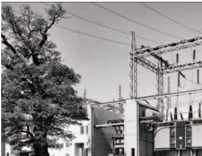
1a The world's largest transformer in 1942 (220 kV / 120 MVA) Värtan substation Stockholm, delivered by ASEA
