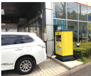
Quick charger installed in a dealer
