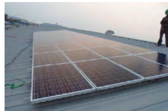
Photovoltaic power generation panels
