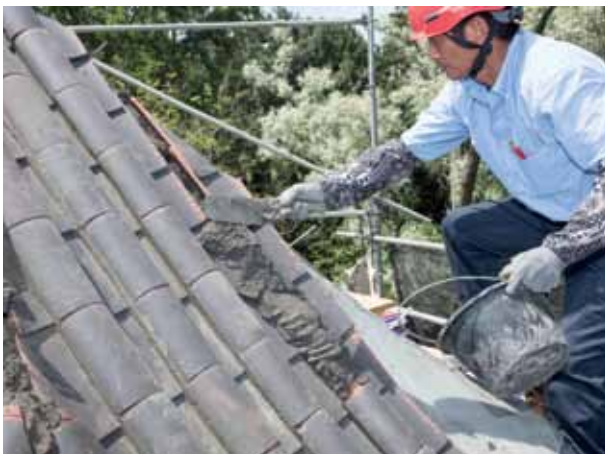
ON THE TOP. The surface of the roof was made from PLANITOP 12 SR. ABOVE. The tiles were bonded to the roof with MAPECEM 202.
