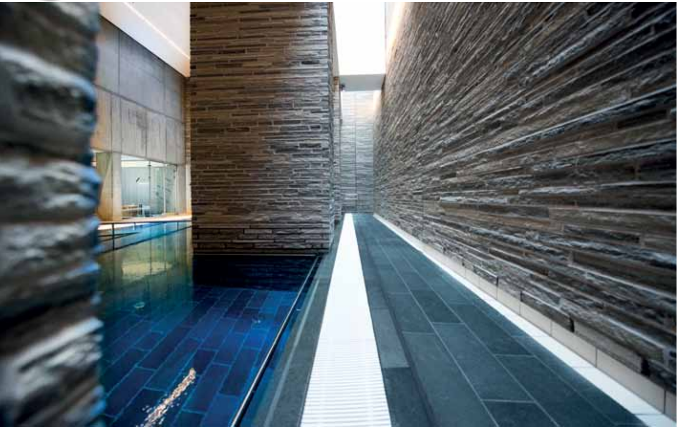
ABOVE. The grout lines were filled with KERACOLOR GG and the joints were sealed with MAPESIL LM and MAPESIL AC.
