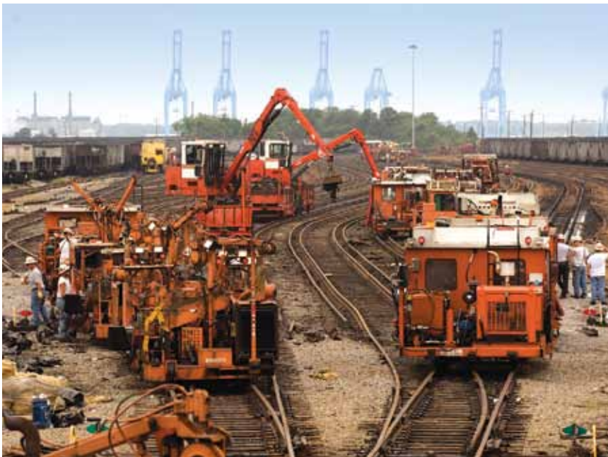
■ Members of a track gang in Norfolk make safety their first priority.
