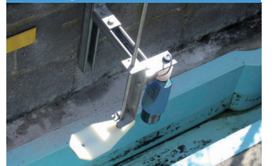
3107 Open channel flow
