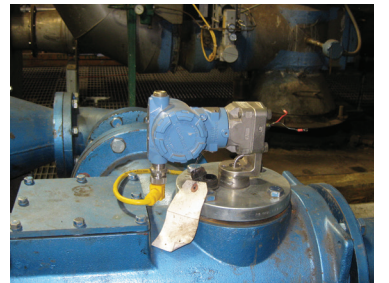
2051 Sludge pump pressure
