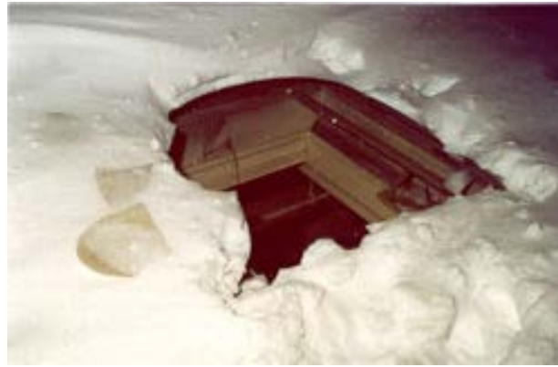
Figure 1. This picture shows the broken skylight where victim fell.
