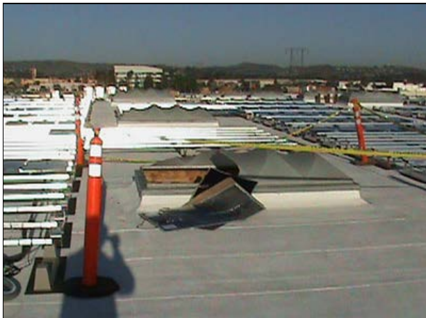
Exhibit 5. A view of the incident scene and the base foundations for the solar panels.
