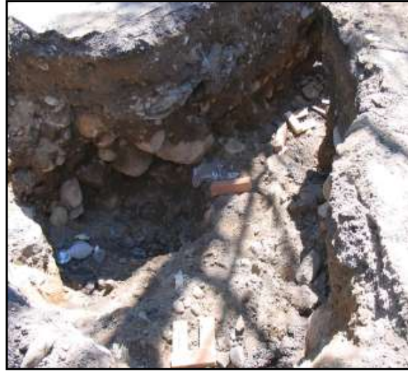
Figure 4: Area of trench collapse Note the large boulders hanging from the excavation faces and undermined areas on the edge of the trench (courtesy of OSHA)
