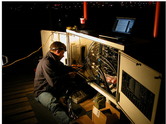
Figure 10. This system installation is configured with solid outer conductor cables. Maintenance activities are usually scheduled to avoid peak operational periods.
