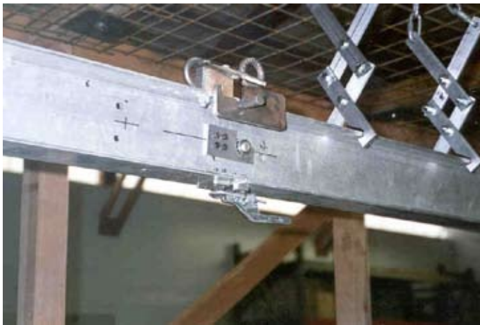
Locking system for aluminum joint sections on in-mine hoist.
