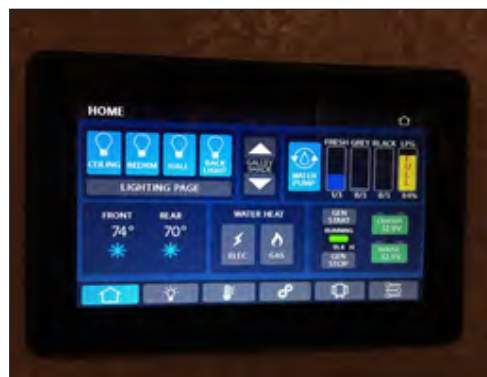
Figure 13-5: Water pump controls
