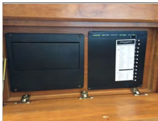
Figure 9-3A: Inside circuit breaker box
