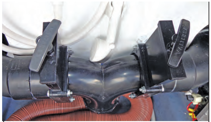
Figure 13-10: Sanitation coupling, valve and hose
