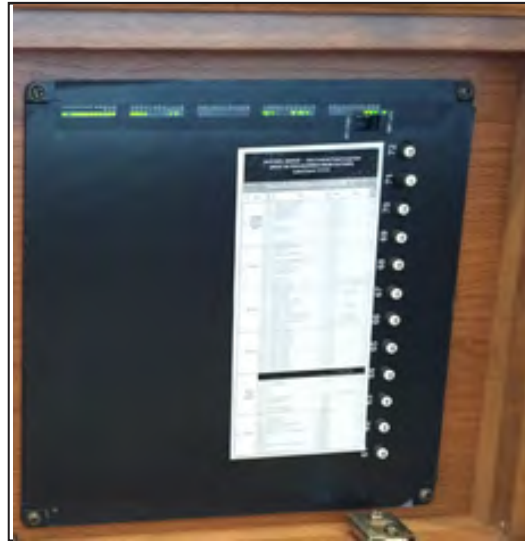
Figure 9-4: Circuit breaker box
