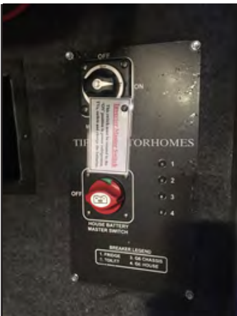
Figure 9-9: House battery disconnect panel
