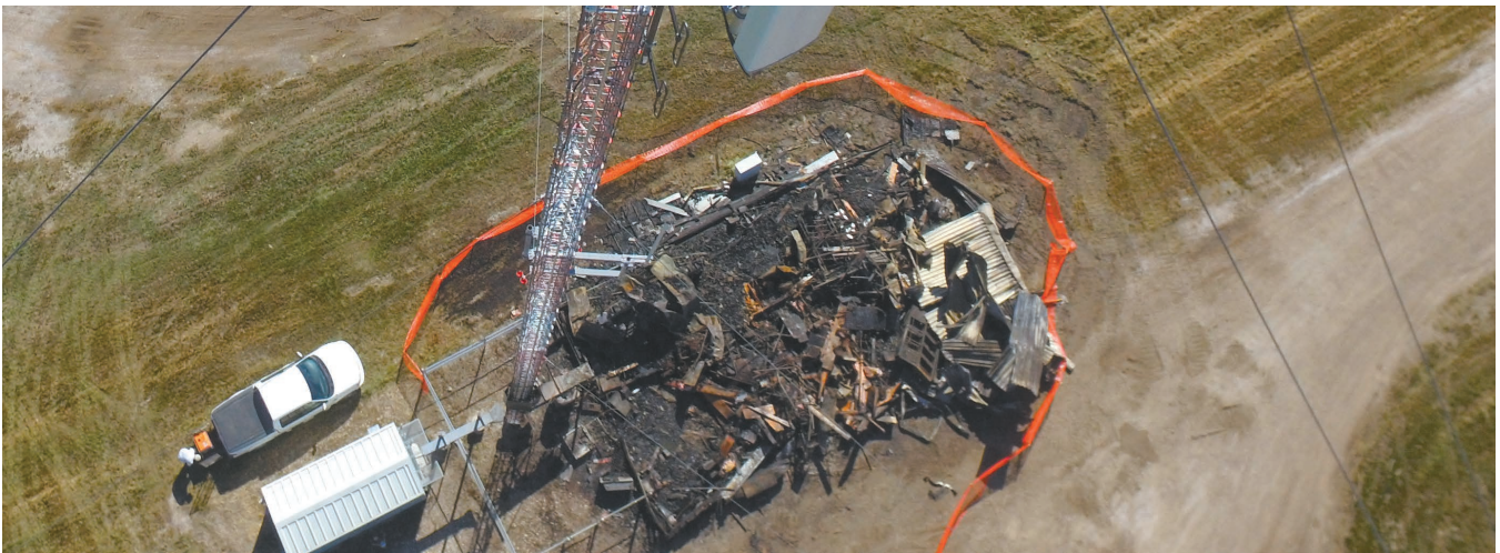
On August 23, 2020, a fire destroyed SaskTel's CO in Spiritwood and SaskTel rose to the challenge of restoring services in the community.
