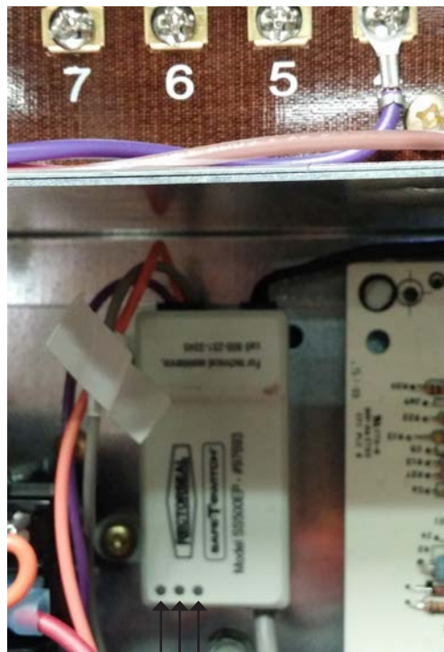
FIGURE 36 Outdoor Condensate Control
