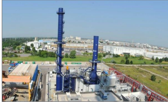
100% Hydrogen GE-10 gas turbine at Enel's Fusina Power Station
