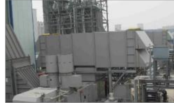
Aeroderivative 2xLM2500 operating on steel mill gases with ~ 58% H 2
