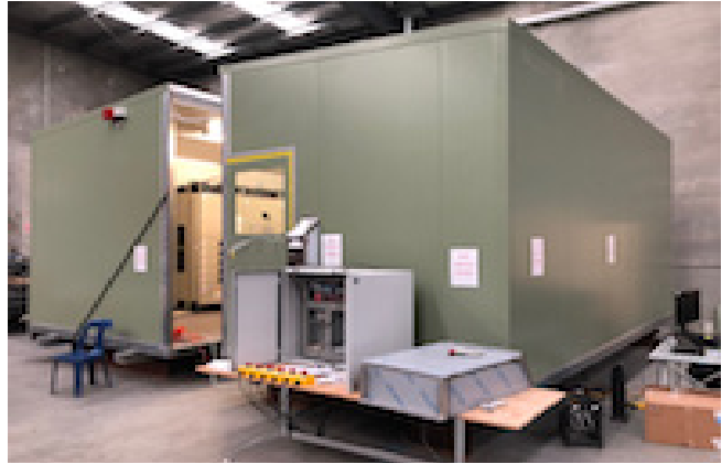
The MCC was pre-built in a portable room prior at SS Electric’s facility prior to being shipped to site
