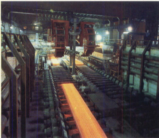
Figure 4: SIMATIC S5-150U programmable controllers from Siemens are installed in this continuous casting plant to control mold adjustment, the dummy bar and cutting length measurement.
