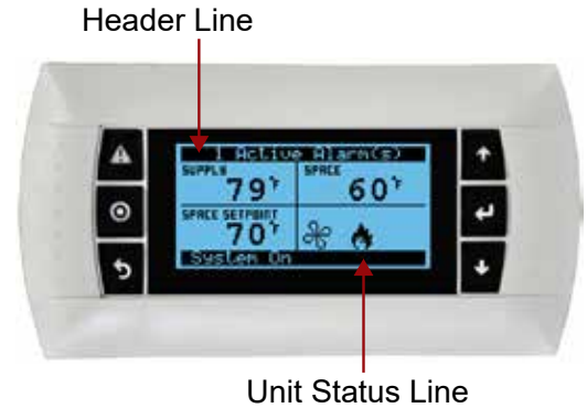
Figure 76: Main Status Screen.
