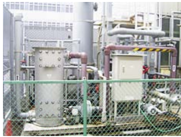
Groundwater purification equipment at the factory at Yamaha headquarters
