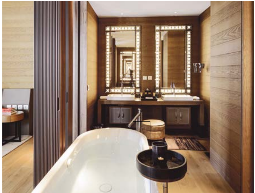
Lengthening of a bath spout for a floor-standing bathtub mixer adapted for the width of the bathtub rim
