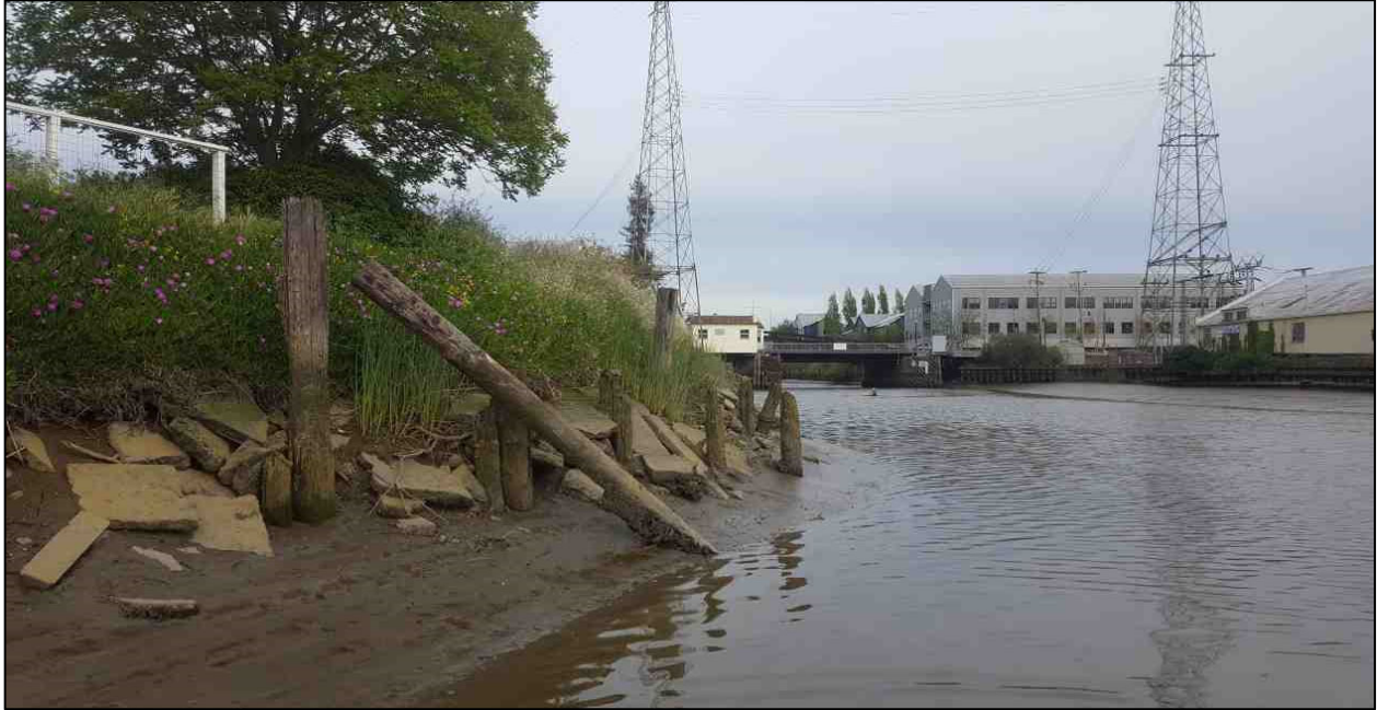
Photograph 1: General location of outlet of storm drain culvert on east bank of Petaluma.
