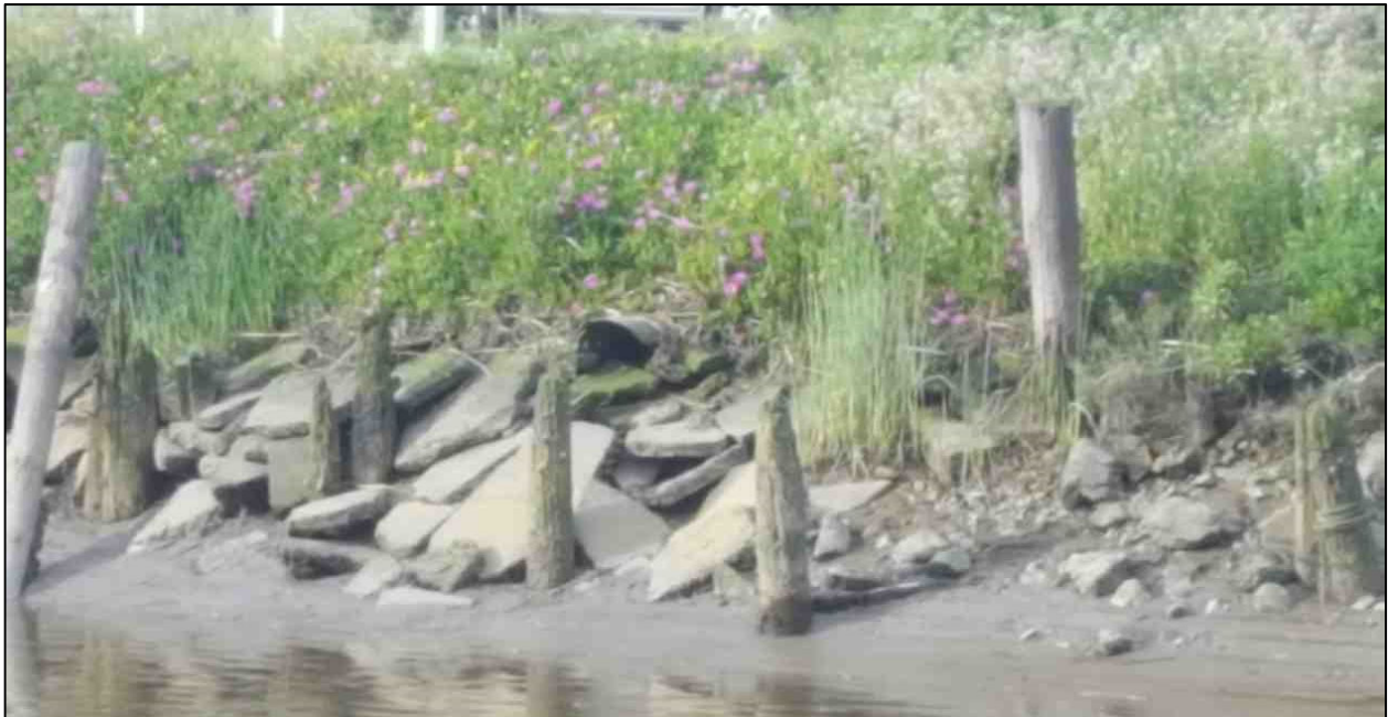
Photograph 2: Outlet of storm drain culvert (photo center) that drains into Petaluma River.
