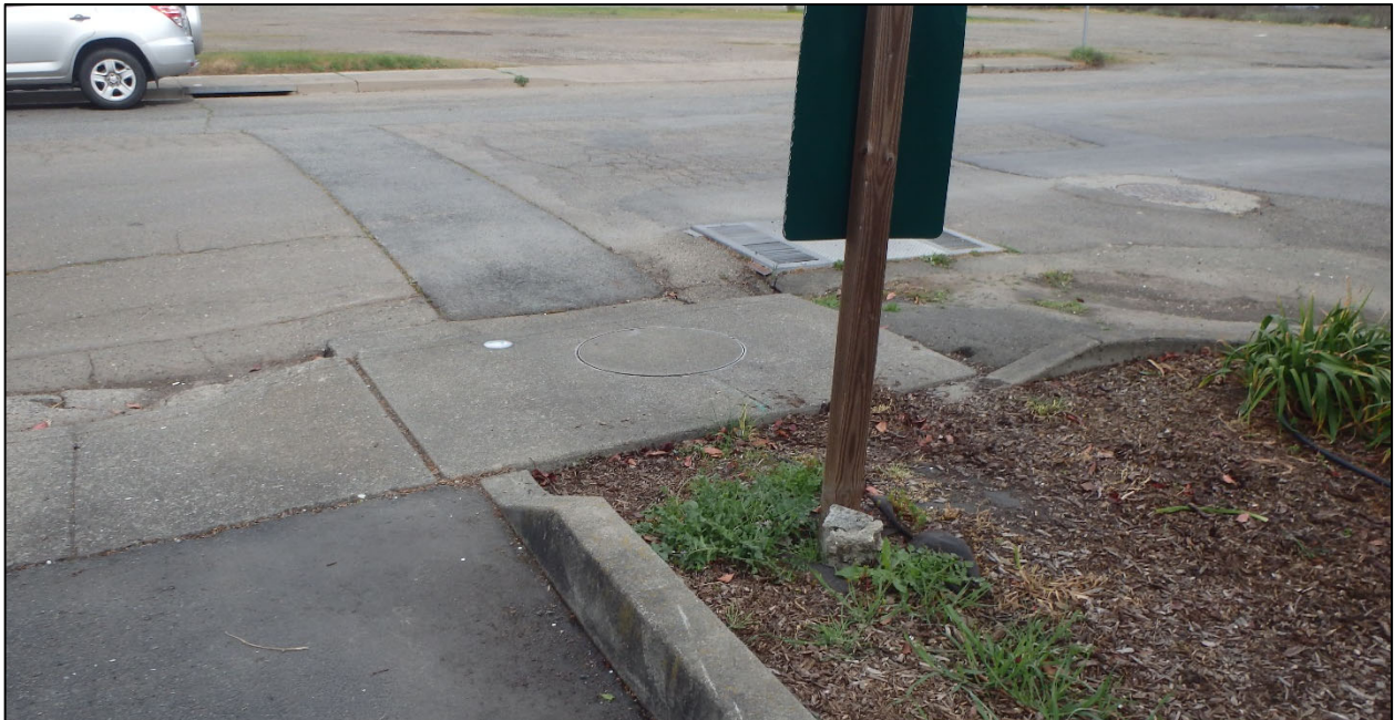
Photograph 8: Curbside storm drain on Weller Street that drains into the existing storm drain which eventually outfalls into the Petaluma River.
