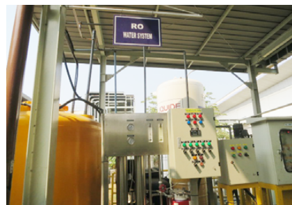
Reverse osmosis membrane equipment
