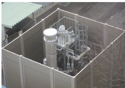
Groundwater purification equipment at the headquarters office
