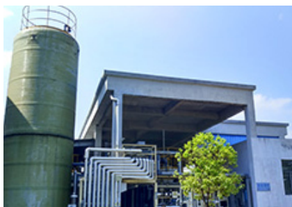
Wastewater treatment facility
