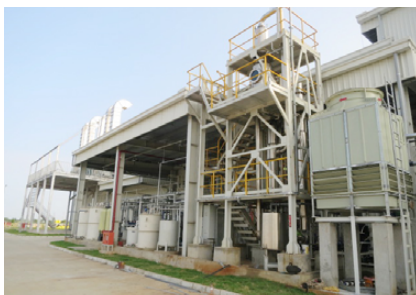
Wastewater treatment facility
