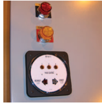
Special Meters and Relays
