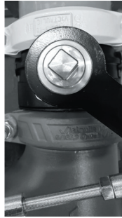
Valve Stem Position – Bypass Valve
