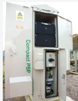
UPS and remote monitoring
