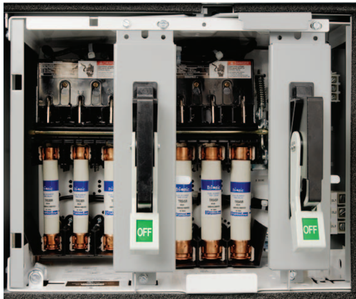
Example of Dual Feeder Disconnect Switch (DFDS)
