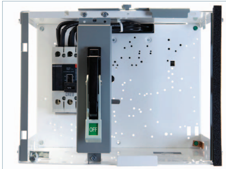
Example of Feeder Circuit Breaker (FCB)
