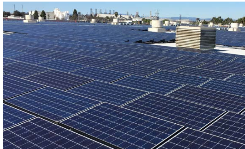
Honda installed one of Southern California's largest corporate owned on-site solar arrays.
