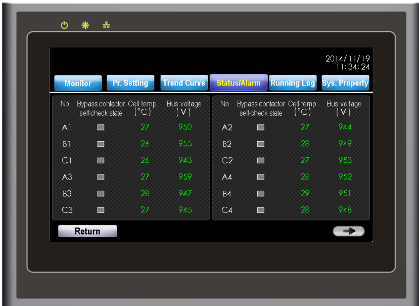
Figure 6-19 Viewing the auxiliary state of power cells
