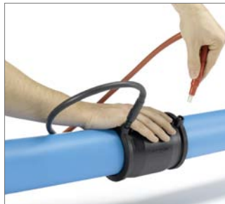
Fig. 47 9. Connect the welding unit; red cable to the red contact. The welding parameters are automatically detected.
