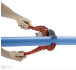
Fig. 39 1. Trim the pipe to the desired length, smoothly and at a right angle.
