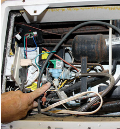
The water valve for the icemaker sits in a harsh environment and is often overlooked during inspection. Plastic lines on the inlet and outlet are susceptible to becoming brittle from heat and cold.
