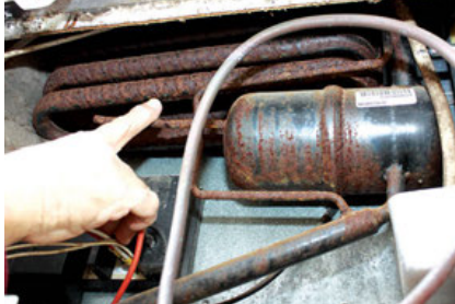
Excess rust will likely cause an early failure of this cooling unit.
