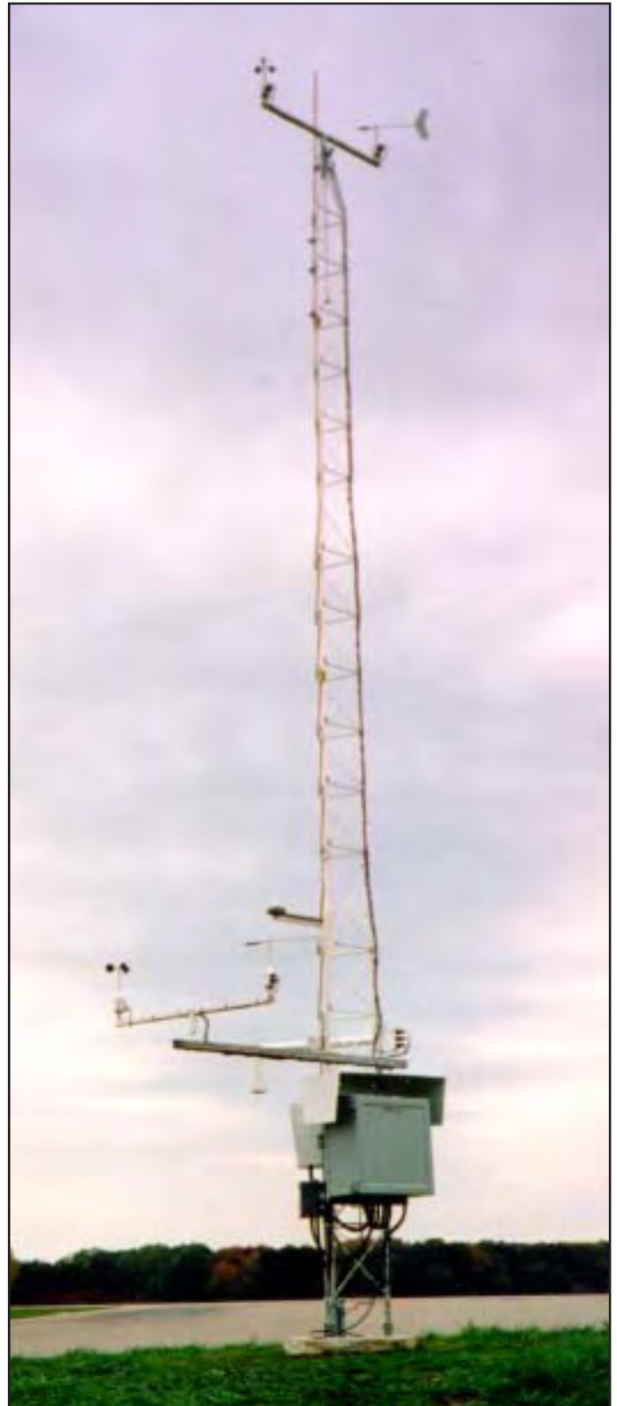
Tower-Mounted Meteorological Monitoring System
