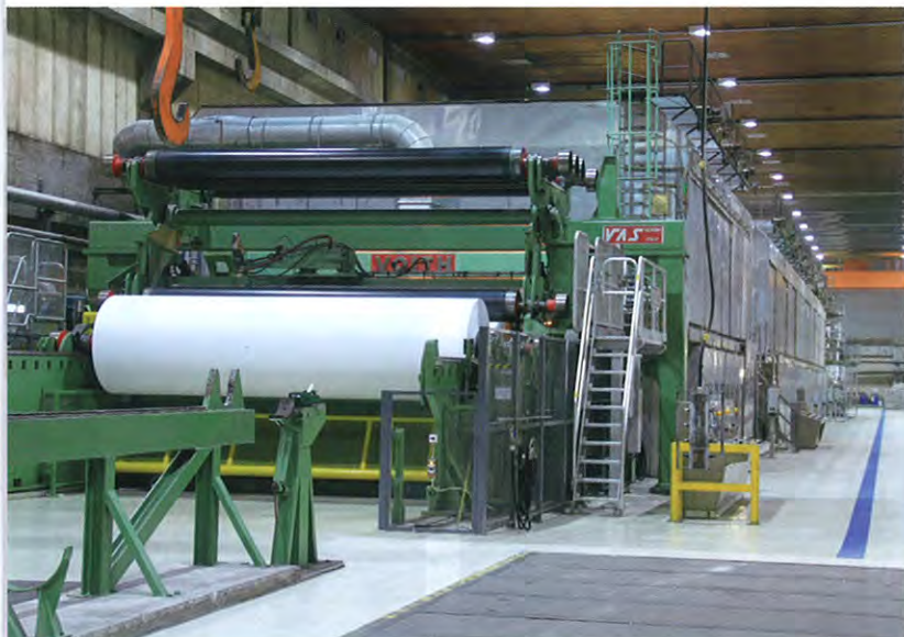
PM 2 is now running with new drives
