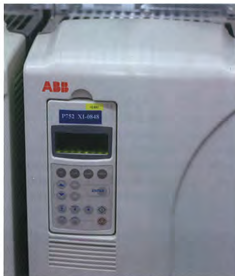
ABB Drive control at Stockstadt
